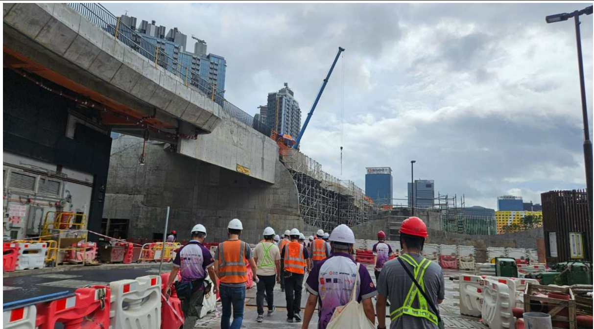
Photo 3: Regular site inspection was carried out to audit the implementation of mitigation measures on site.
